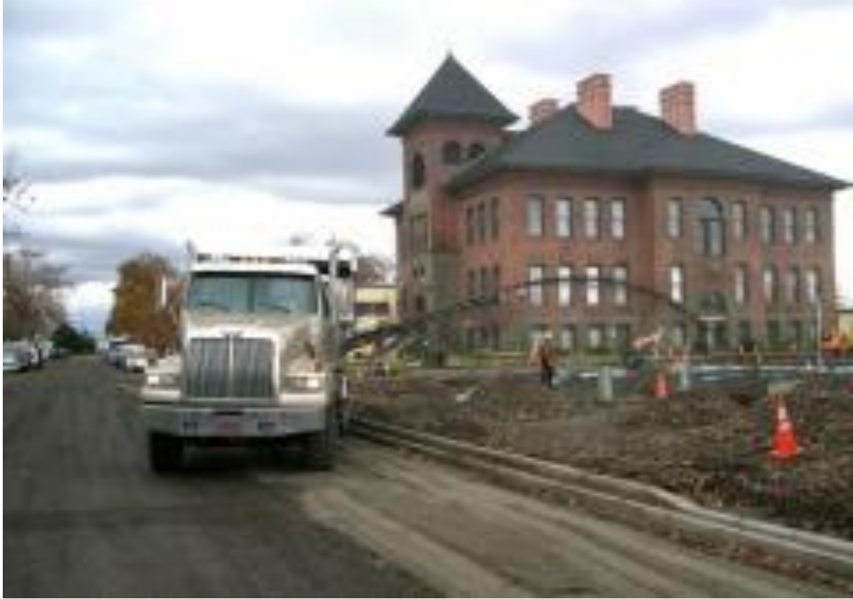
Figure 2 — A Stone Slinger “throw conveyor” throws aggregate through the air at a construction site. Stone Slinger is a trademark of W.K. Dahms Mfg. Ltd. (Photograph used with permission. For more information, www.stoneslinger.com )
