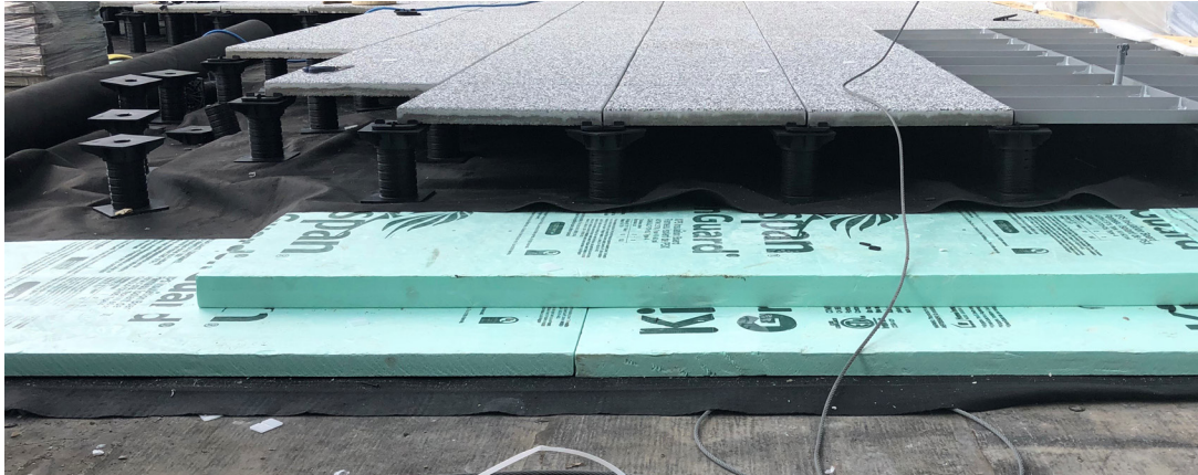
Figure 1 — This Protected Membrane Roofing Assembly features a moisture barrier covered with multiple layers of XPS insulation, in turn topped with a fabric covering and finished with spacers and a layer of paving material. Photo courtesy of Kingspan.
