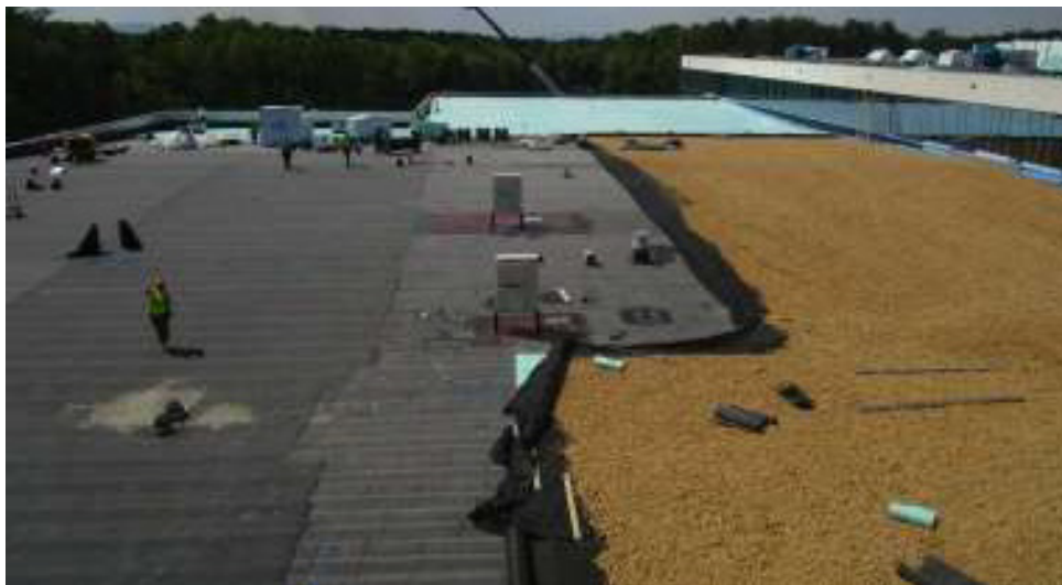
Figure 2 — A basic PMRA consists of a waterproofing membrane, XPS insulation, a fabric covering and aggregate for ballast. This PMRA is for a federal building in Winchester, Virginia. The distributor was Carlisle Coatings & Waterproofing. The installer was Kalkreuth Roofing & Sheet Metal. Photo Courtesy of Kingspan.
