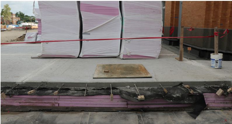
Figure 1 — XPS insulation used with a split slab configuration as part of a Protected Membrane Roof Assembly on Dickies Arena in Fort Worth, Texas. Note how the roof covering is protected by the insulation. Photograph taken during construction, courtesy of Owens Corning.
