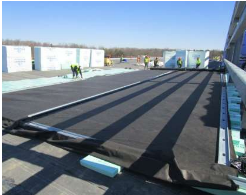
Figure 5. The PMRA is in process of being covered with aggregate shortly after the XPS insulation boards are covered with fabric. The aggregate not only holds the insulation in place but also reflects sunlight from this PMRA, which is in a warm humid climate zone. Photo Courtesy of Kingspan.
