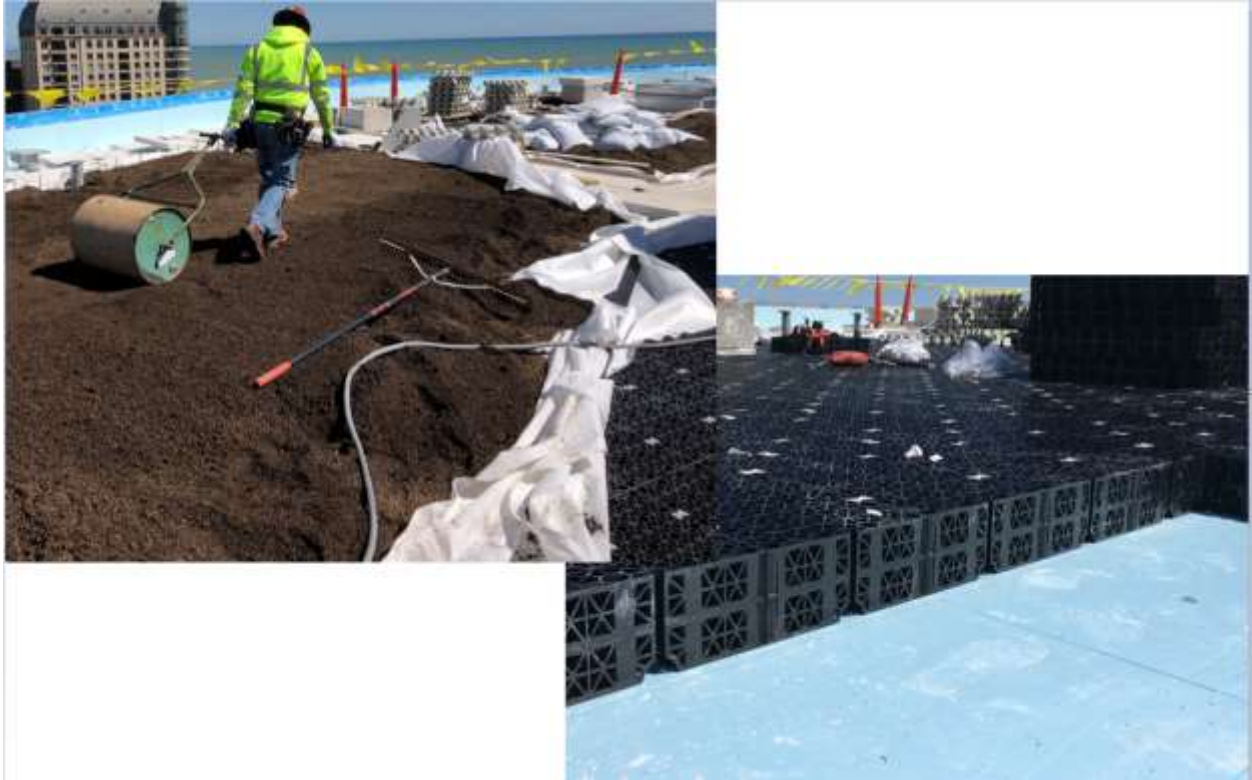
Figure 8. The key to this blue roof is a sturdy water storage unit located above the XPS insulation and just below the vegetative roof assembly. Photos Courtesy of American Hydrotech.
