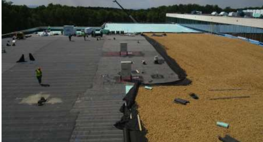
Figure 3. A basic PMRA consists of a waterproofing membrane, XPS insulation, a fabric covering and aggregate for ballast. This PMRA is for a federal building in Winchester, Virginia. The distributor was Carlisle Coatings & Waterproofing. The installer was Kalkreuth Roofing & Sheet Metal. Photo Courtesy of Kingspan.
