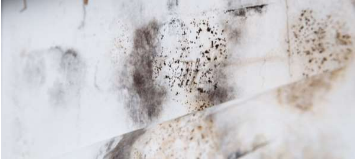
Figure 6: If basement walls are not insulated from the outside, the wall temperature could drop below the dew point. Moisture condensation in the dark spaces behind interior insulation and sheet rock creates conditions that favor the growth of mold and mildew. (Abohe Stock)
