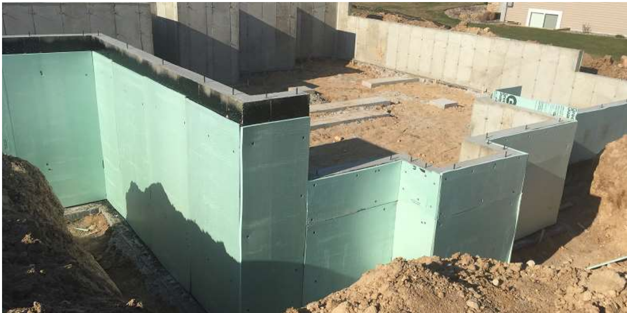
Figure 2: Exterior insulation and damp-proofing or waterproofing along with effective drainage helps prevent water intrusion into the basement. (Courtesy of Kingspan.)
