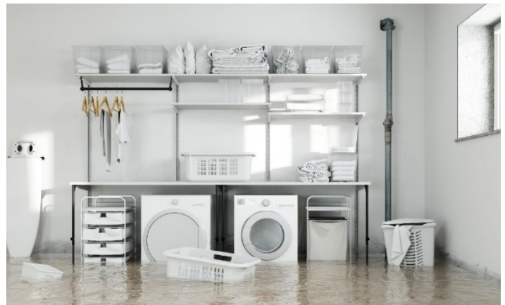
Figure 2: This basement has a water management problem. A habitable basement must have effective environmental separation, meaning bulk water must not penetrate the interior of the basement. (Adobe Stock)
