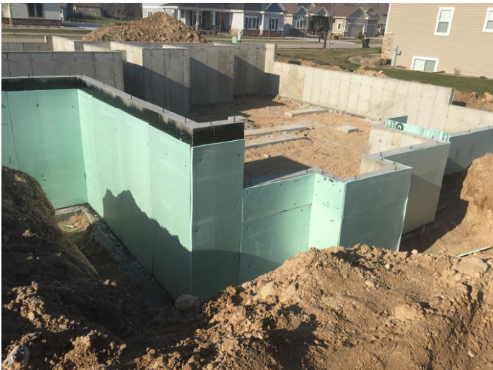
Figure 1: Exterior insulation and damp-proofing or waterproofing along with effective drainage helps prevent water intrusion into the basement. (Courtesy of Kingspan.)
