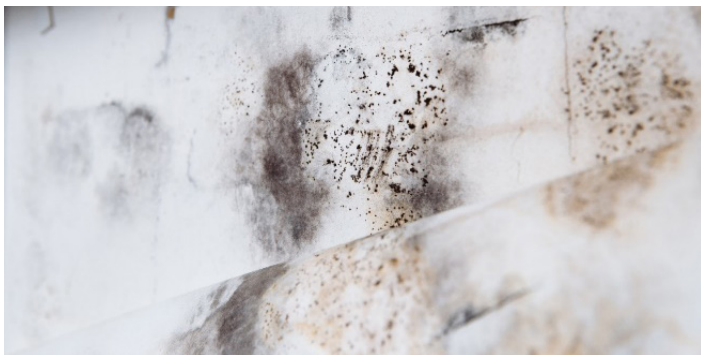
Figure 1: If basement walls are not insulated from the outside, the wall temperature could drop below the dew point. Moisture condensation in the dark spaces behind interior insulation and sheet rock creates conditions that favor the growth of mold and mildew. (Adobe Stock)
