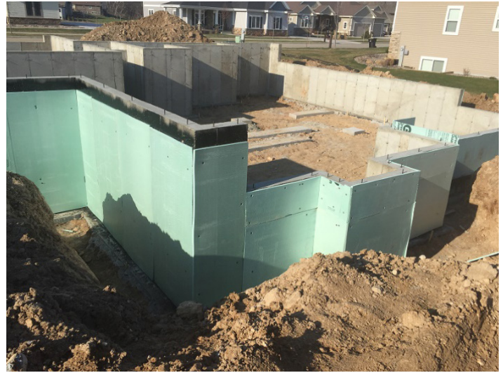
Figure 4: Exterior insulation and damp-proofing or waterproofing along with effective drainage helps prevent water intrusion into the basement. (Courtesy of Kingspan.)
