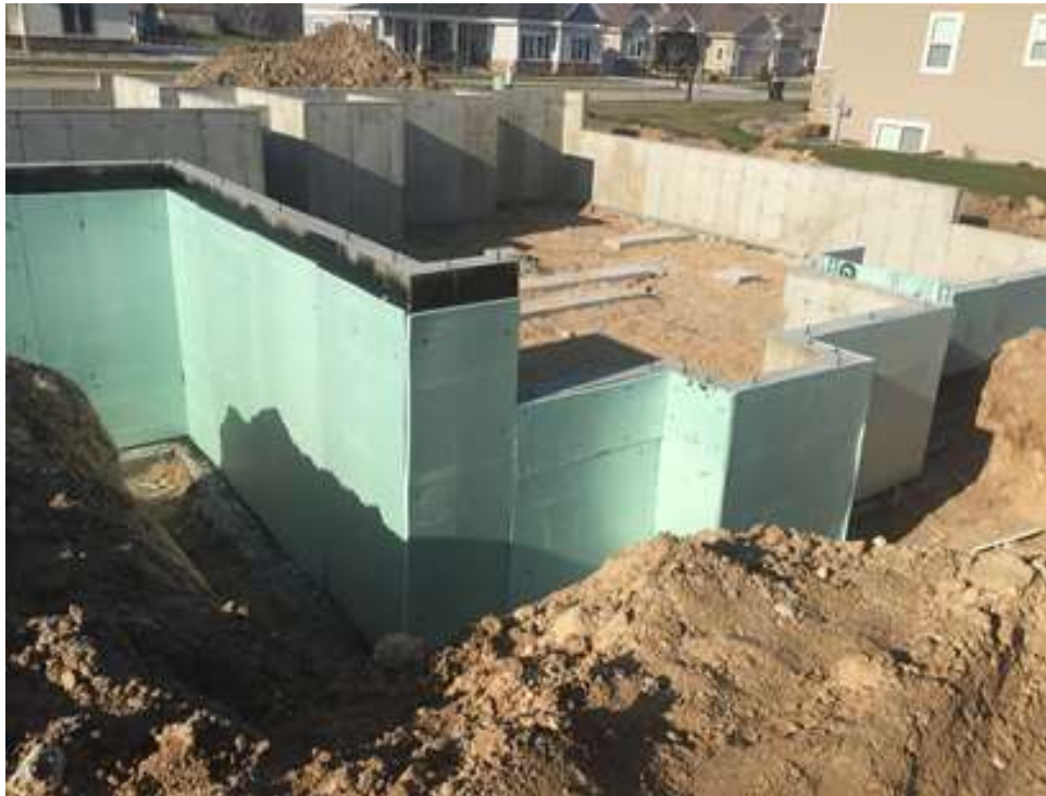
Figure 2 — RCPS is often installed in below grade applications for habitable basements. (Photograph Courtesy of Kingspan.)
