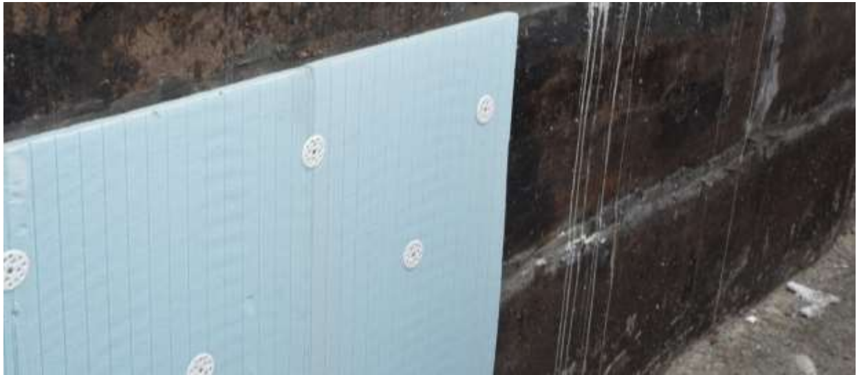
Figure 9: XPS insulation on exterior of basement wall showing damp-proofing, wall insulation and anchors outdoors. (Adobe Stock)
